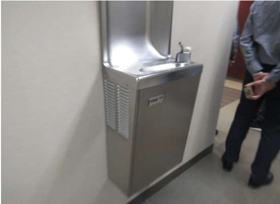
5th floor hallway drinking fountain not Operating properly
