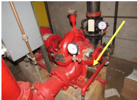
Basement fire pump water leak dripping
