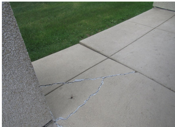
Sidewalk cracks and sunken suggests a potential compacting/stability issue
