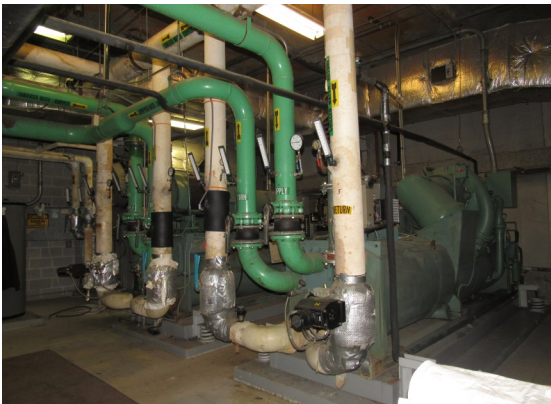
View of main Chiller system that appear to be 1978 original build—past repairs noted
