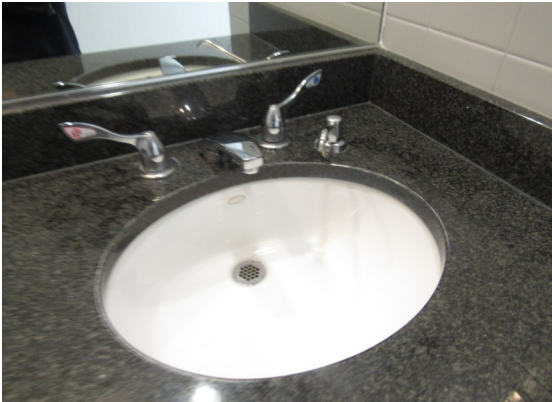
4th floor Mens room sink has dripping faucet
