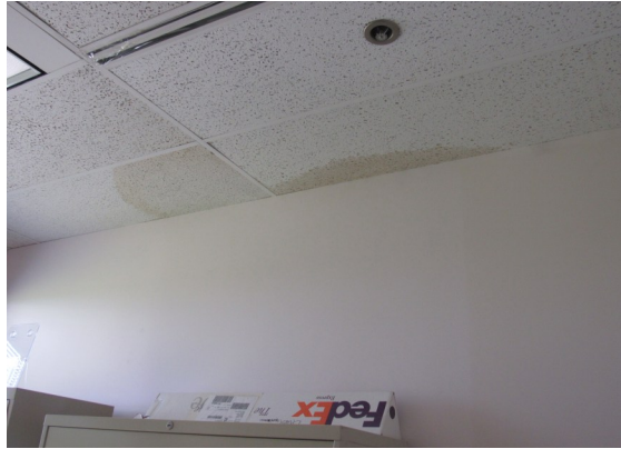
Multiple ceiling stains on 5th floor
