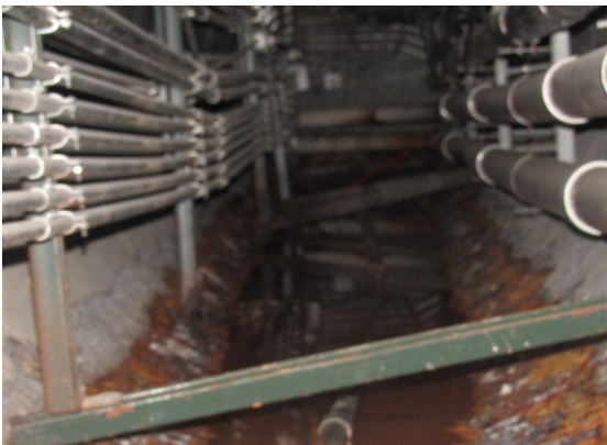
Tunnel water with no apparent drain
