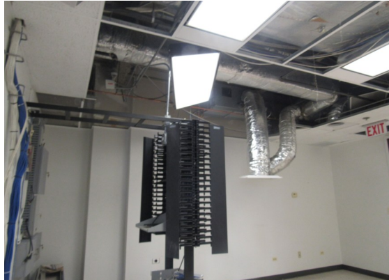
Suite 410 data room abandoned with low voltage and HVAC not fully decommissioned
