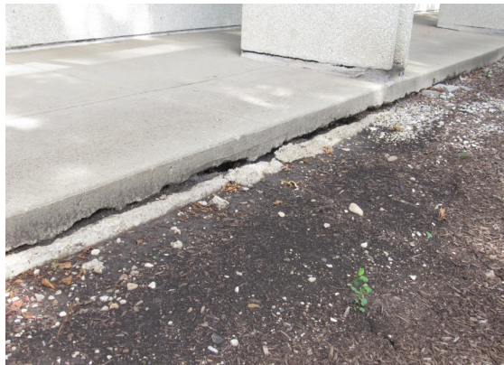
Underpinning erosion at sidewalk landing
