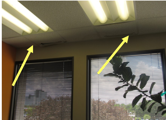
Suite 200 Ceiling, wall and window stains
