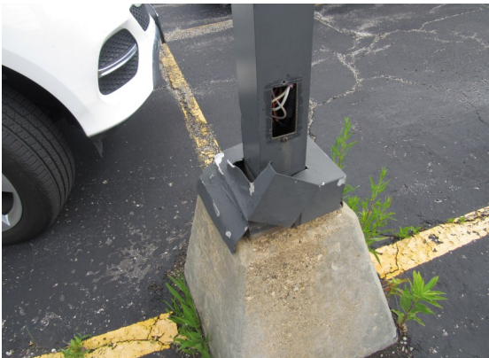
Impact damaged and exposed wiring at Parking lot overhead light
