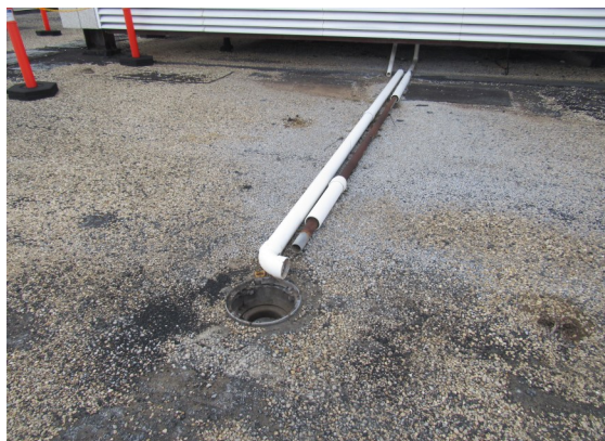
Missing downspout cage screens at roof
