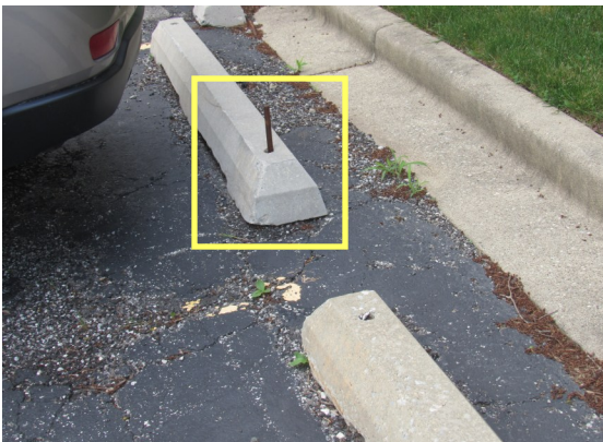
Exposed re-bar at parking blocks is a safety Hazard
