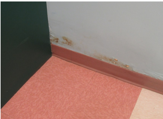
Deli area past water damage on wall
