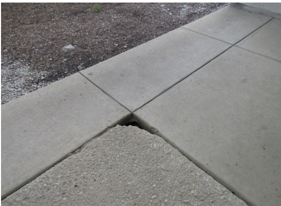
Void / hallow area under the deteriorated sidewalk along the side of the building near the subsurface generator
