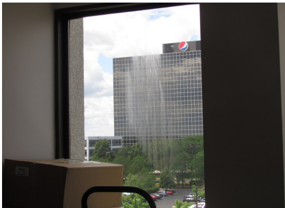
Fogged window example
