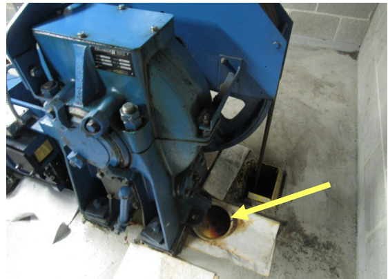
Oil collection at elevator mechanics
