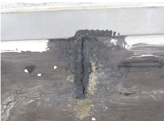
Past patching repairs re-cracking on roof
