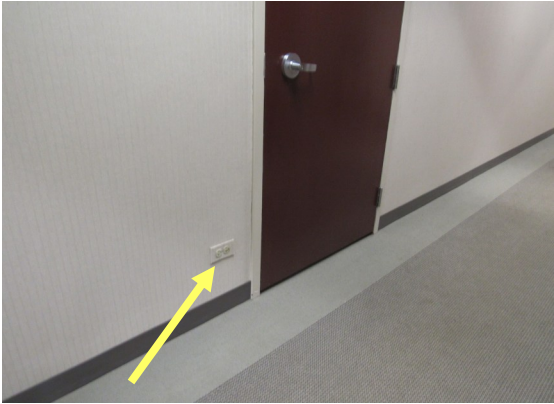
5th floor hallway outlet with broken ground
