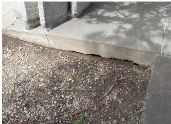
Underpinned sidewalk from drainage erosion
